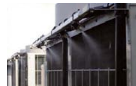
E mizu Shower installed on outdoor air conditioning systems
